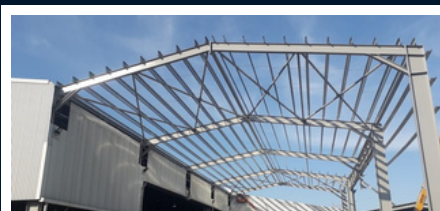
Gas Treatment Plant Warehouse- DUGAS
